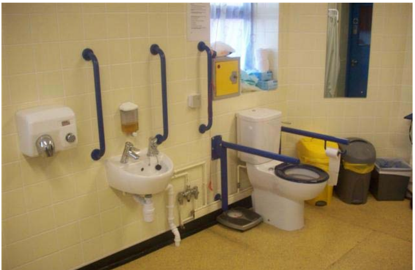
Toilet with space for assistance
